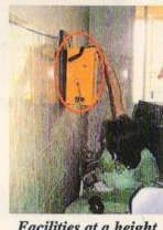
Facilities at a height
